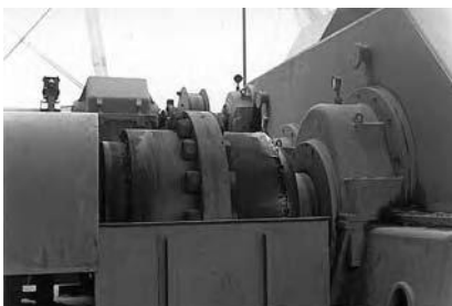
Cement kiln mill drive
